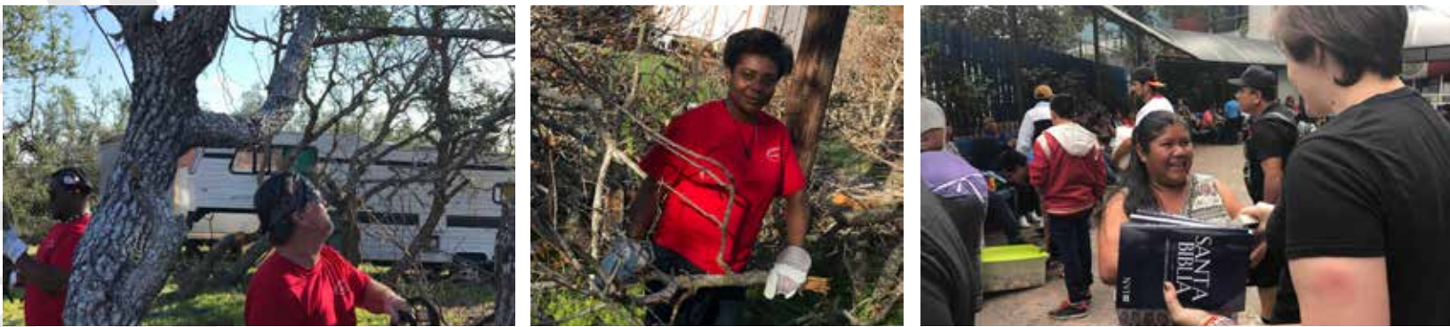
Wilson Kamera, Tim Feazell (left), and Enyo Assoklou (center) remove trees at a trailer park. Right: Charlie Doak, AIMer in Mexico City, hands out Bibles.
